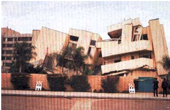
Apartment with soft stories that partially collapsed after the 1994 Northridge earthquake.
